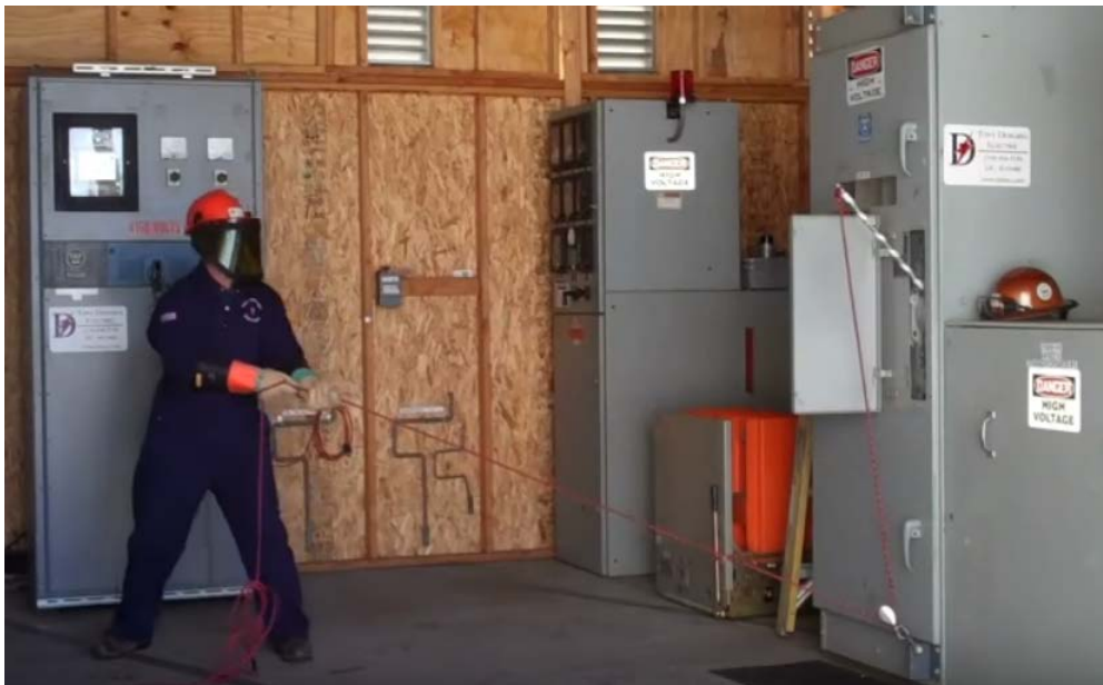
Manual Operation of a Medium Voltage Switch with Rope and Pulleys
