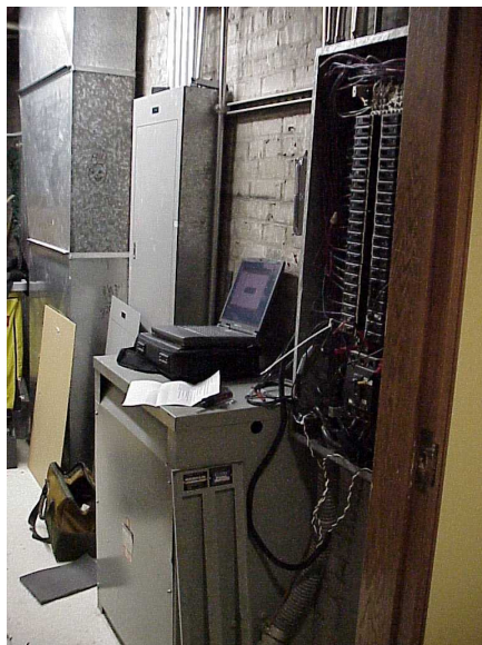
Picture 1 - Electrical Closet, Transformer, and Panelboards
