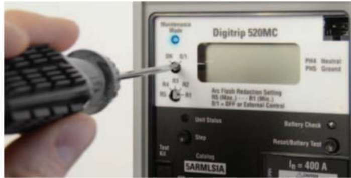
Photo 5 – Arc Flash Reduction Mode on Trip Unit
